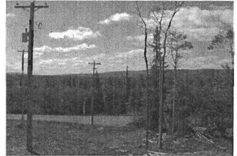
Distribution line from the Stewart Crossing substation to the community
